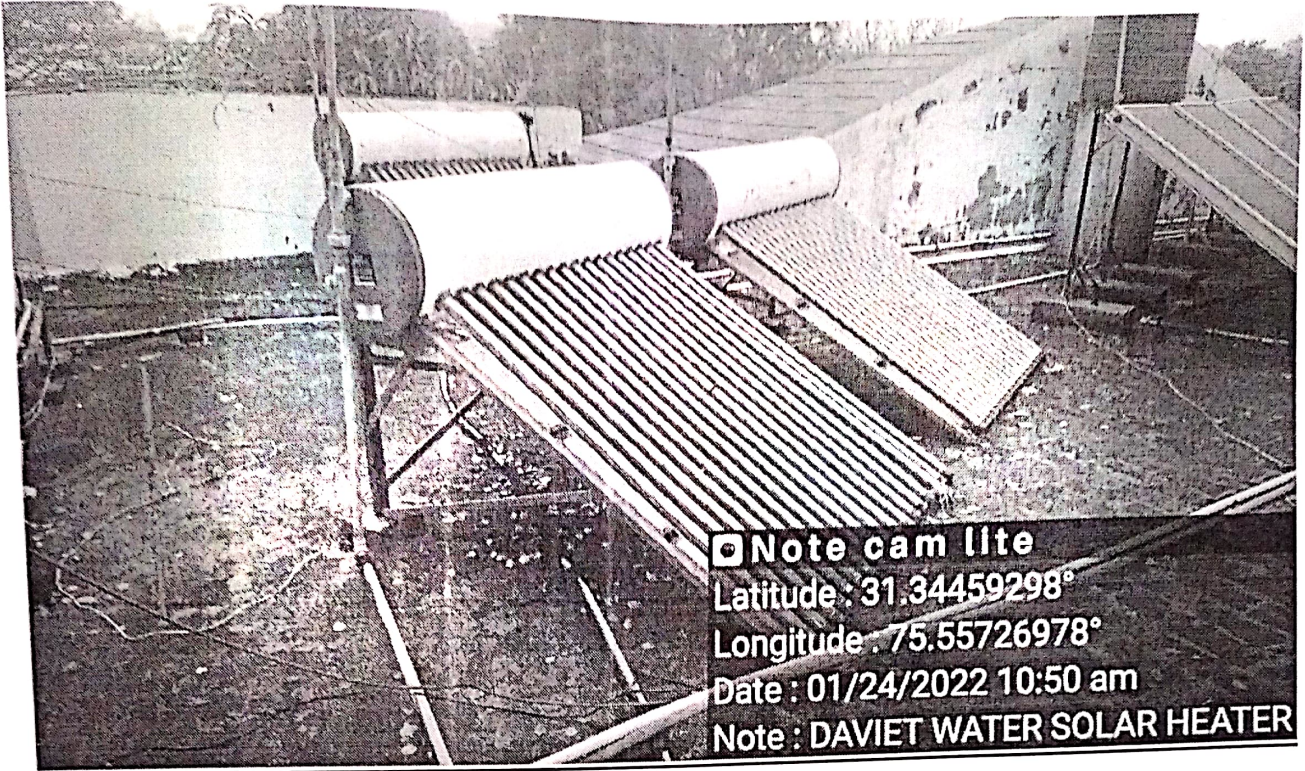
Solar Heater System in the DAVIET campus
