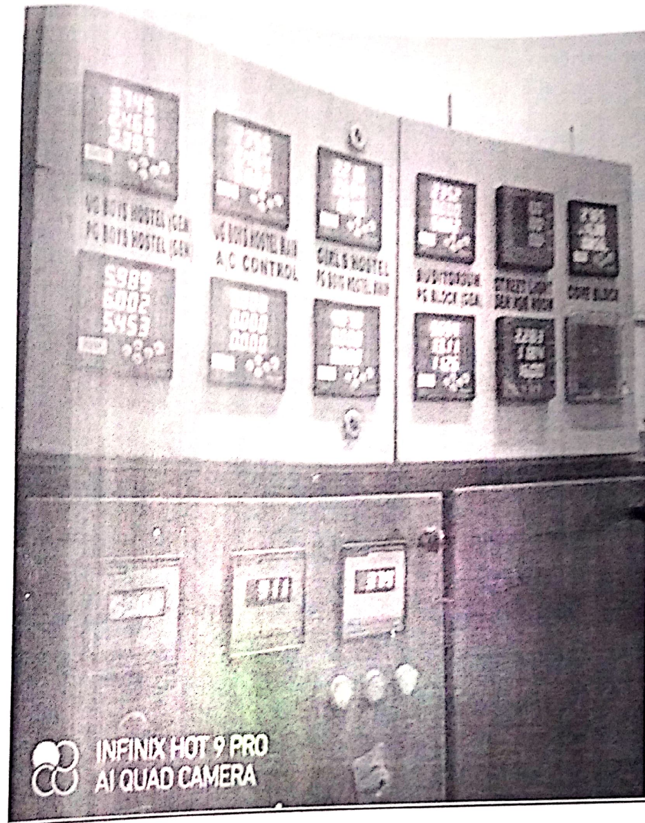
MFM Schneider, Digital meter and CT Current Transfprmaer for the Sensor based energy conservation systems installed in DAVIET, Jalandhar
