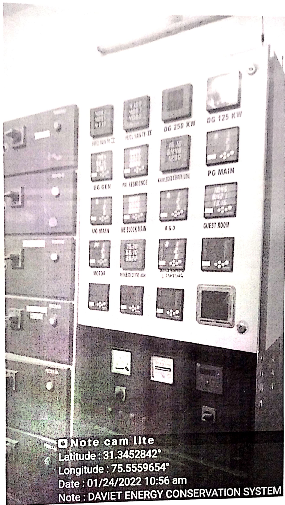
MFM Schneider Smart meter for the Sensor based energy conservation systems (3 no.) installed in DAVIET, Jalandhar
