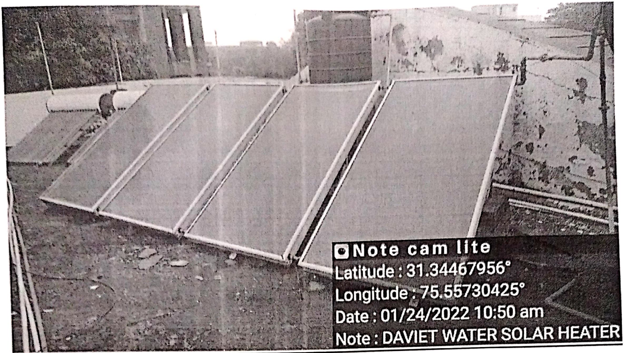
Solar Heater System in the DAVIET campus
