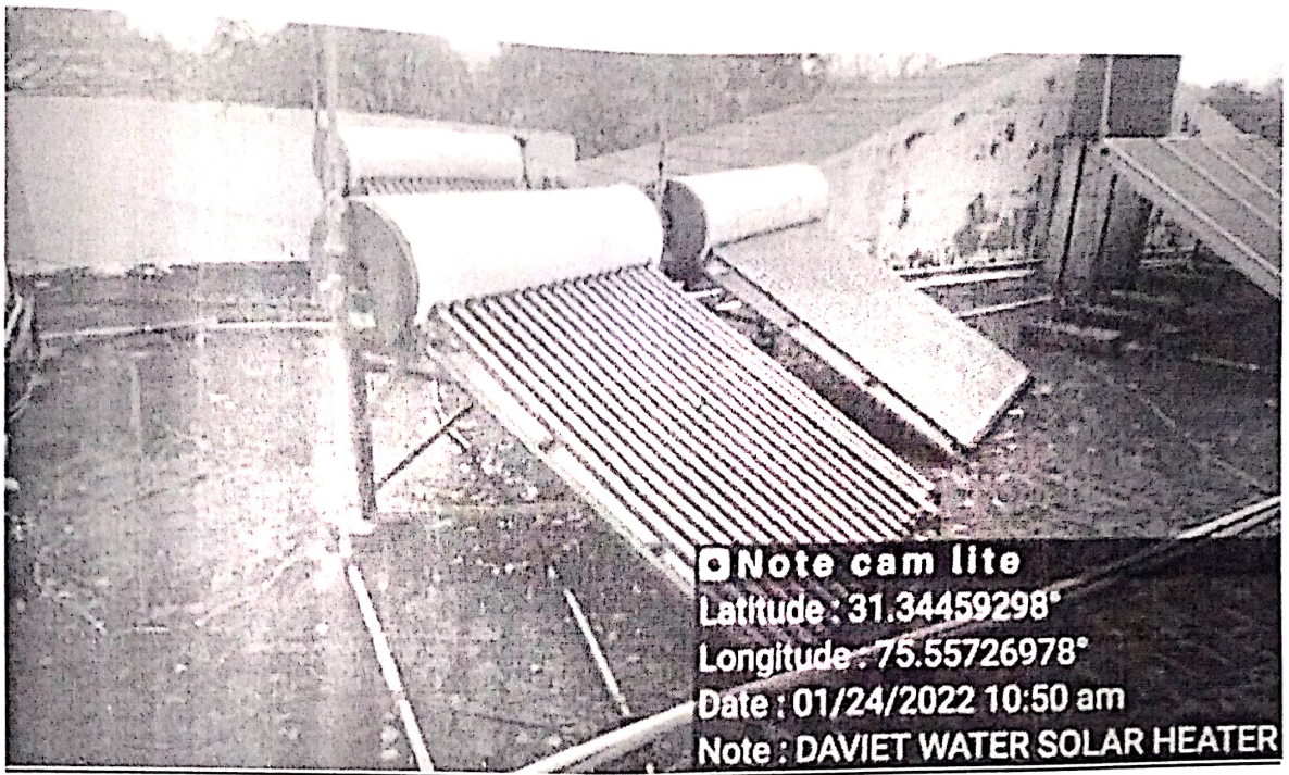
Solar Heater System in the DAVIET campus
