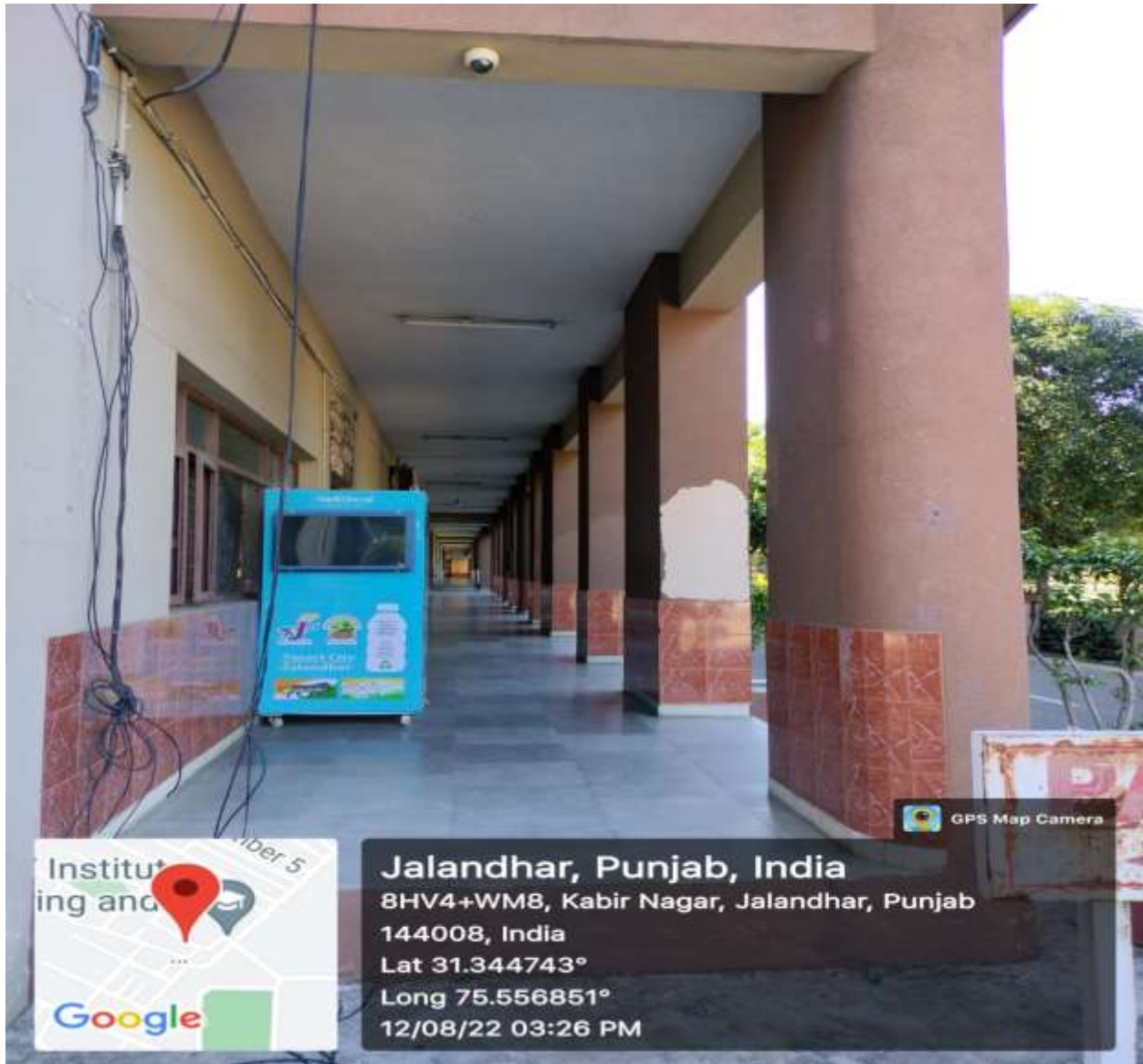
Security Camera in Corridor
