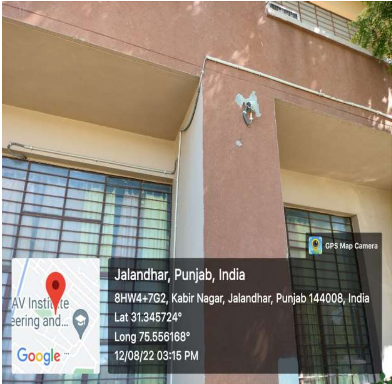
Security Camera in Corridor
