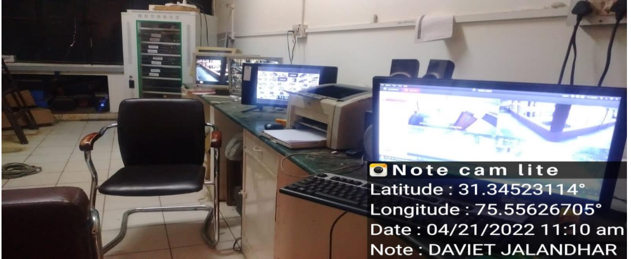
CCTV surveillance Room
